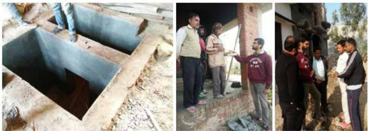
FIGURE 46: SEPTIC TANK WITH INCORRECT DESIGN AT A HOUSEHOLD CONSTRUCTION SITE AND CONSULTATION WITH LOCAL MASONS
