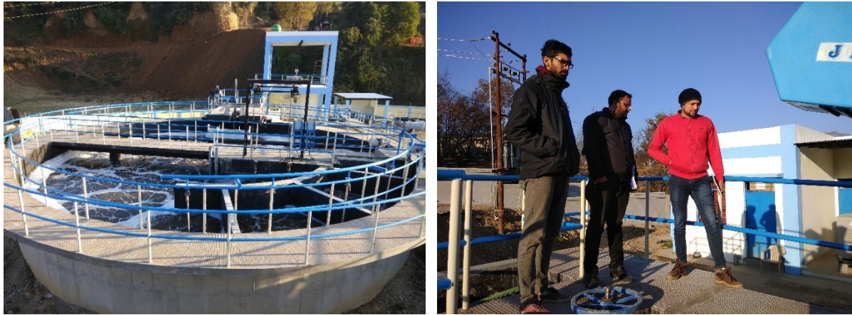
FIGURE 55: SEWAGE TREATMENT PLANT AT NIRADA, PITHORAGARH (1.25 MLD CAPACITY)
