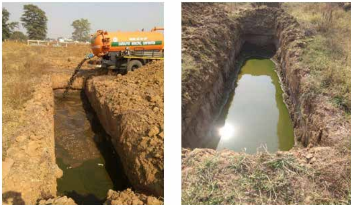
FIGURE 75: DEEP ROW ENTRENCHMENT BEING PRACTICED FOR SAFE DISPOSAL OF SEPTAGE (SOURCE: OWSSB, ODISHA)
